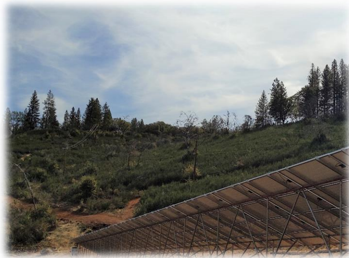
Solar panels on the NCSA property
